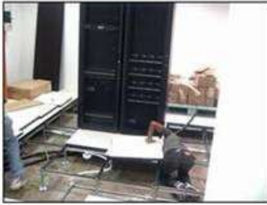
80KVA UPS installation Durban
